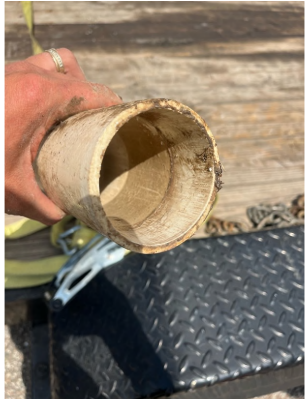
Leak under Clyne Field was the result of no glue
